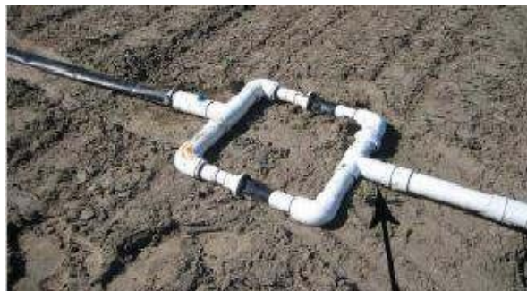
Figure: Pressure regulators installed side-by-side allow a greater flow rate.
